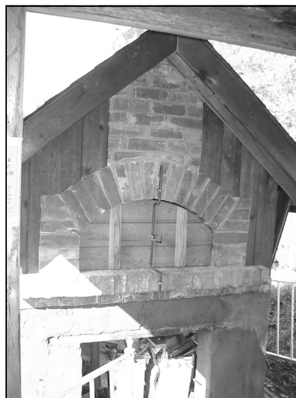
Right: The completed oven with the lockable outer door in place. This door was handcrafted by a local woodworker and a blacksmith.
