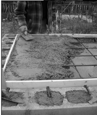
Left: Finally, the concrete is smoothed over the rebar frame to finish the slab.
