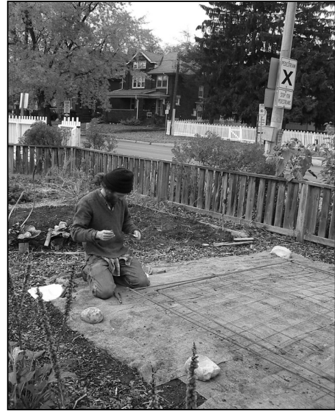
Above: Second, on the side prepare the rebar and mesh. Lay this grid on the insulation sheets before the concrete is poured. This will reinforce the concrete slab base.
