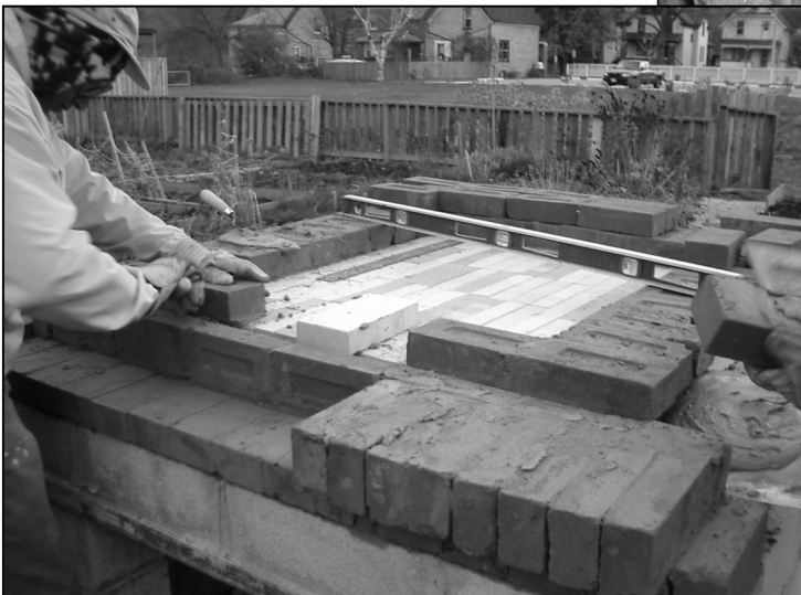
Left: Laying the first course of the red clay brick oven wall!
