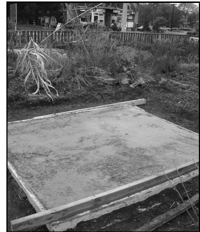
Above: Fourth, the freshly poured concrete slab is smoothed over using an old 2x6 piece of lumber.
