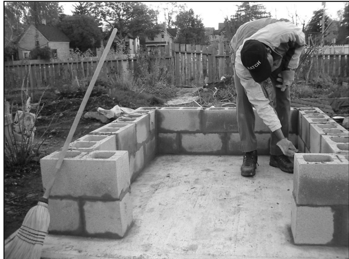
Above: Remember to clean any excess mortar off the bricks before it has time to dry. This can be done by sweeping with a broom or wiping with a damp cloth.
