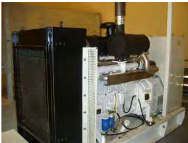
One of three 100kW dutch generators at Garalo able to run on Jatropha oil, diesel or a blend (Photo: Smail Khennas)
